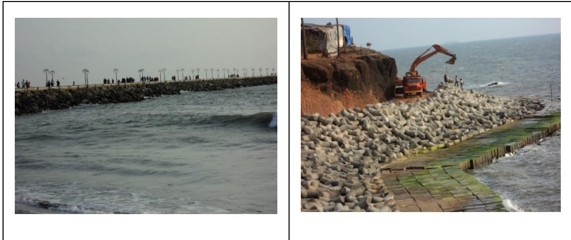
Figure 2.14 (a) Rip Rap around a sea promontory in Kozhikode and (b) Tripods made of concrete in Goa, laid along wave fronts to prevent erosion.
